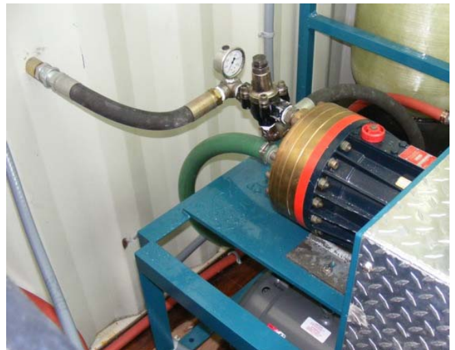
Demucker installed in CES Unit.
