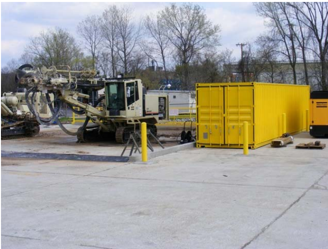
Self-Contained Unit (CES) On-Site at Large Equipment Company.
