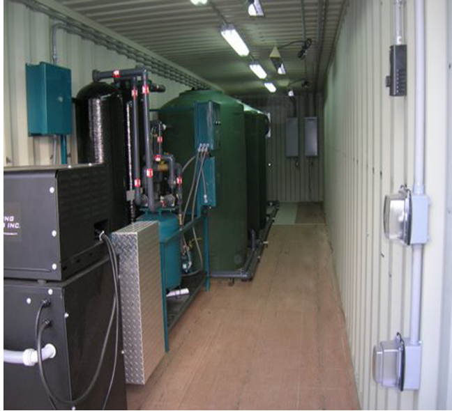
Inside view of Equipment Container
